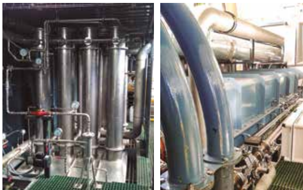
HYDRAULIC CO-GENERATION SYSTEM IN WATER ABDUCTION AND DISTRIBUTION NETWORK (HYGENET) _LIFE12 ENV/ES/000695
